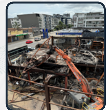
Asbestos fire Makesafe Canterbury
