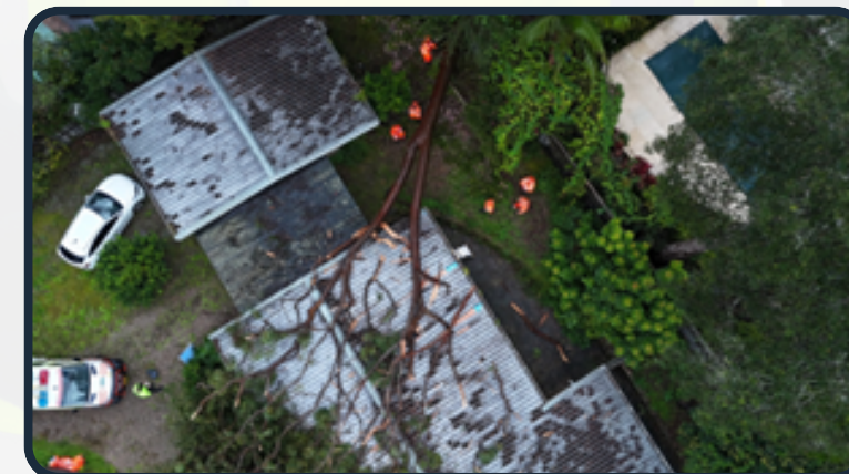
Tree damage Makesafe Cairns
